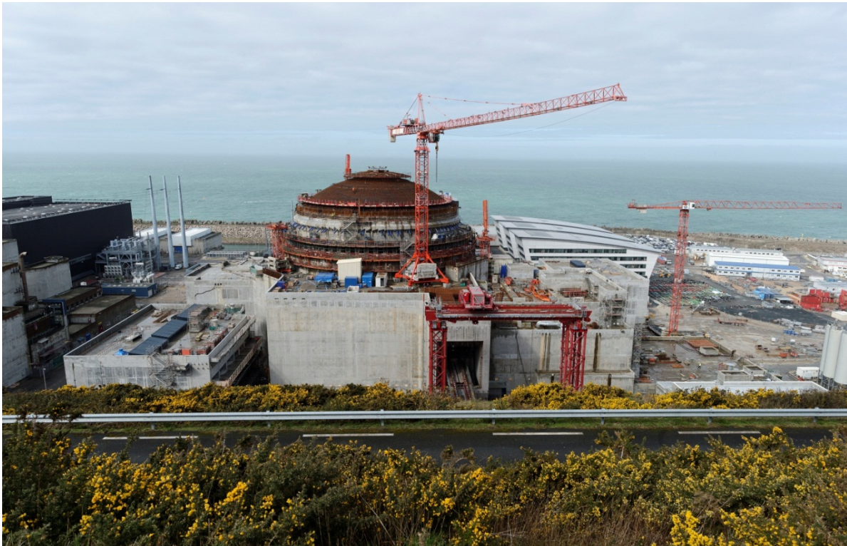
Flamanville 3 – Construction site from the hill, EPR, France, 24 March 2015 (© EDF Médiathèque Alexis Morin – Antoine Soubigou/All rights reserved. Aménagement Flamanville 3, Communication).
