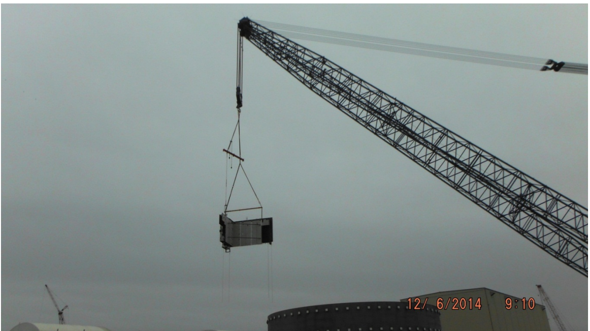
V.C. Summer Unit 2 – Installation of 180k-Pound CA05 Module, AP1000, United States, 6 December 2014 (SCE&G, all right reserved).
