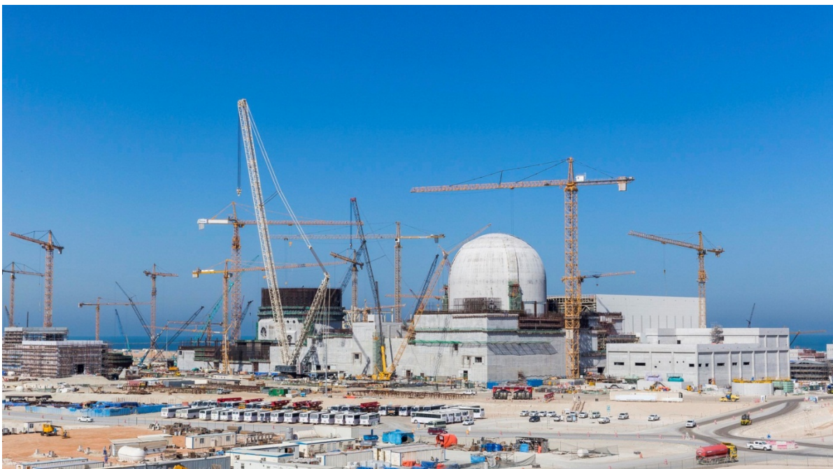
Barakah Unit 1, 2 and 3 – Overview of the construction site, APR1400, United Arab Emirates, 3 February 2015 (property of ENEC).
