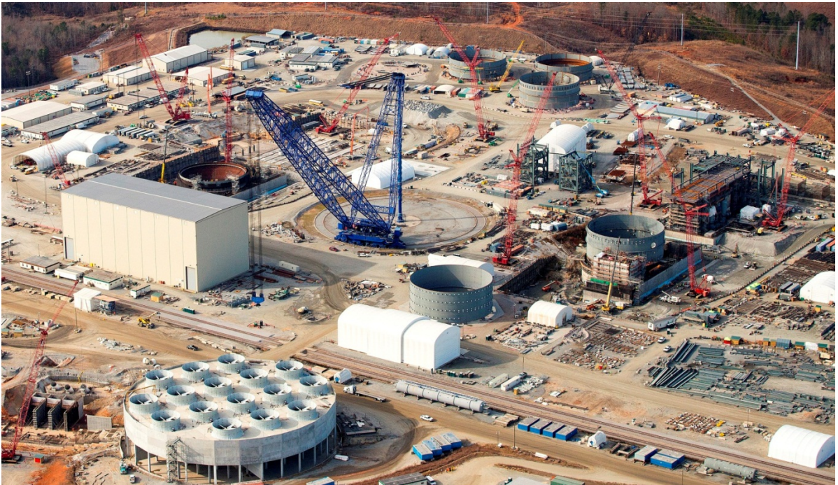
V.C. Summer – Units 2 and 3 nuclear construction project, AP1000, United States, December 2014 (SCE&G, all right reserved).
