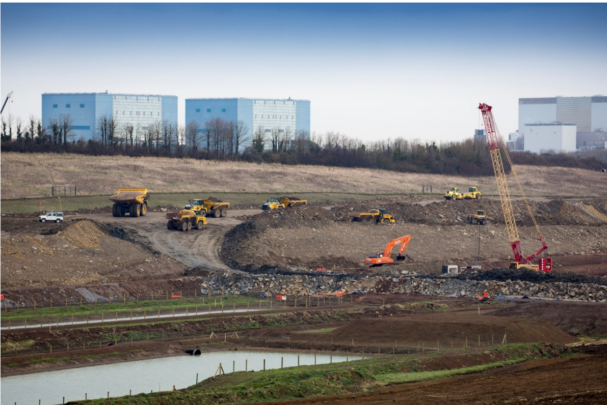
Hinkley Point C – Formation of the southern heavy haul road and construction of the Holford Culvert, EPR, United Kingdom, January 2015 (© EDF Energy 2015).
