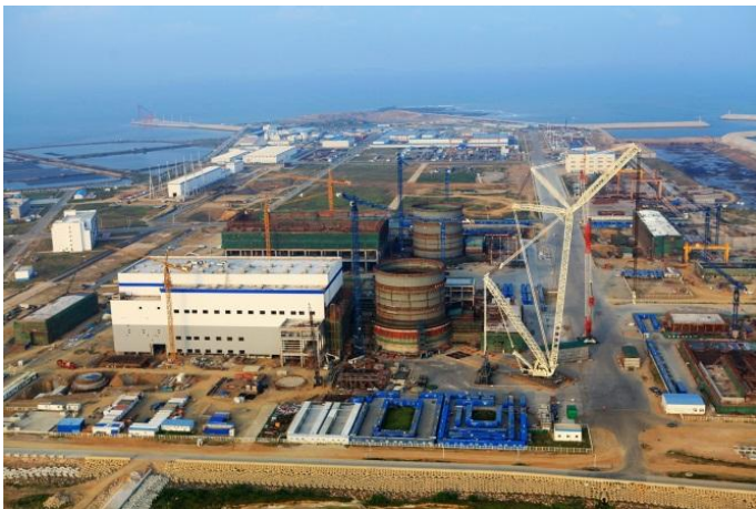
Haiyang AP1000 reactors, China.
