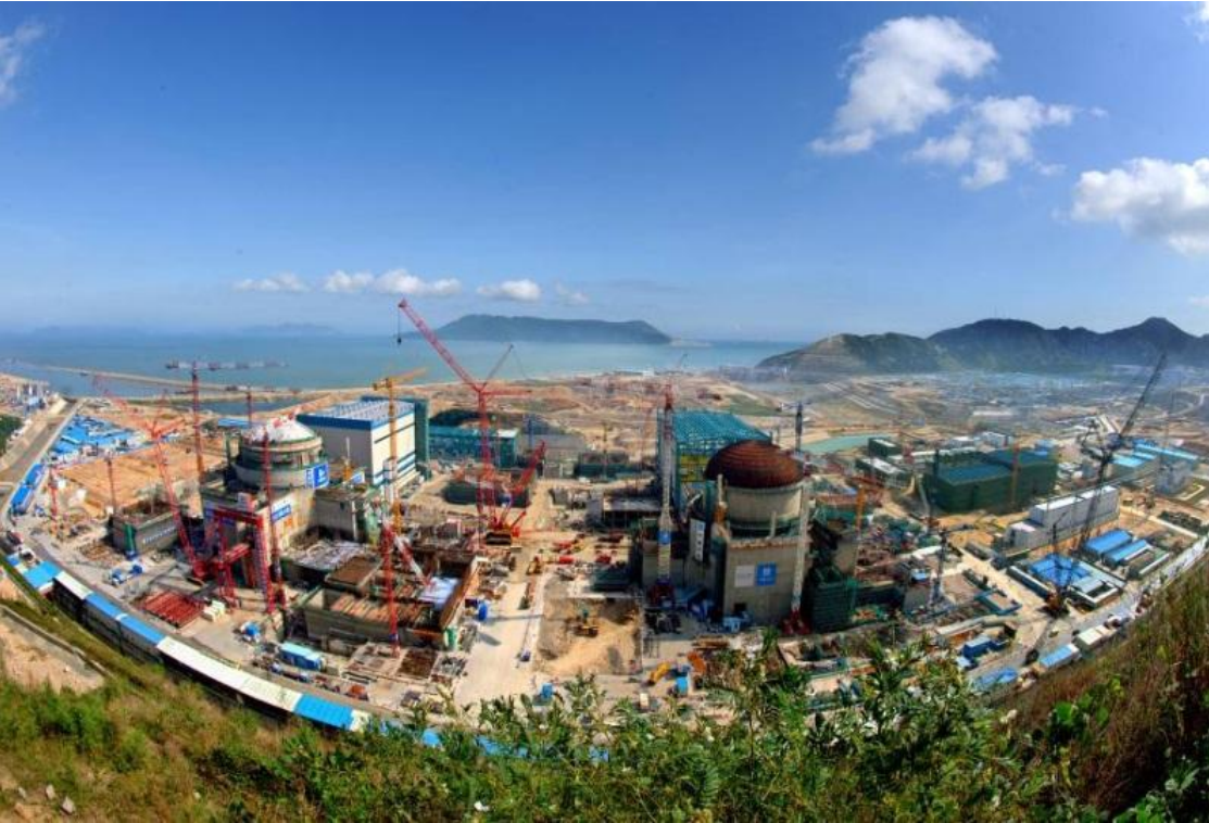
Taishan EPR reactors, China.
