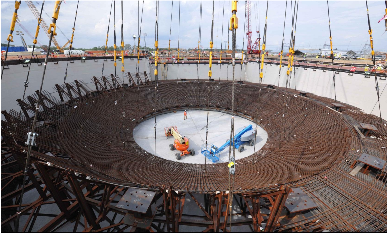
The 460-ton Vogtle Unit 3 CR10 "cradle" is placed into the nuclear island, marking the first major lift of the Vogtle 3 and 4 project.
