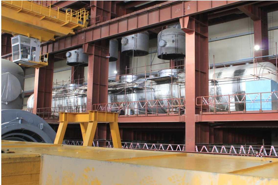
Novovoronezh VVER reactor, steam generator, Russia: 2013. Provided by Rostekhnadzor
